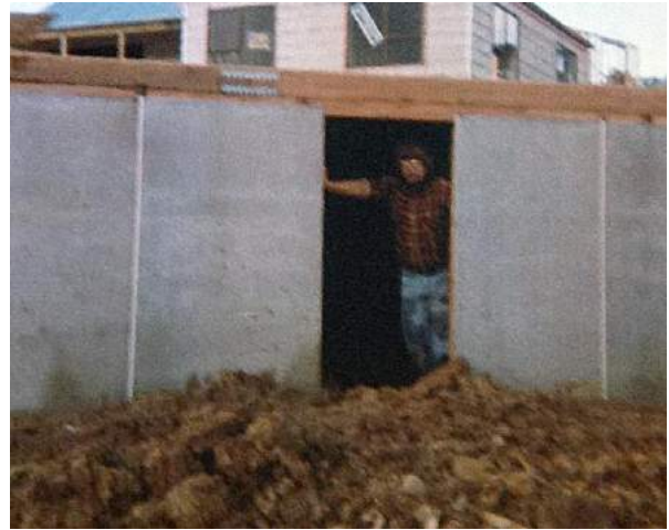
I spent weeks (day and night) up to my knees in mud during the construction
